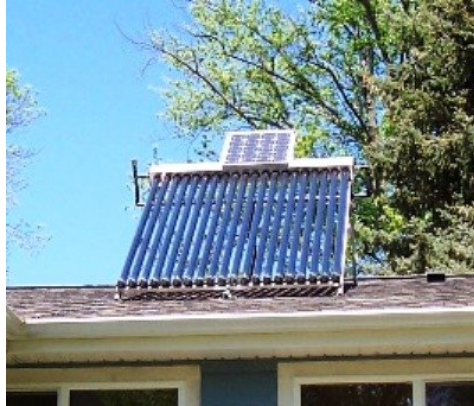
Solar Thermal Collector
