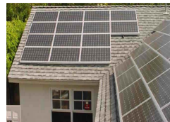
Solar PV panels on roof.
